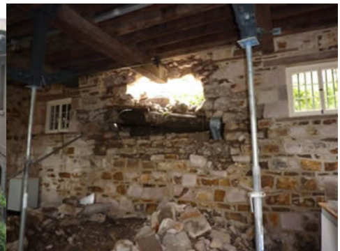
Damage to Old Commissariat Store (photo by Ruth Kerr)
