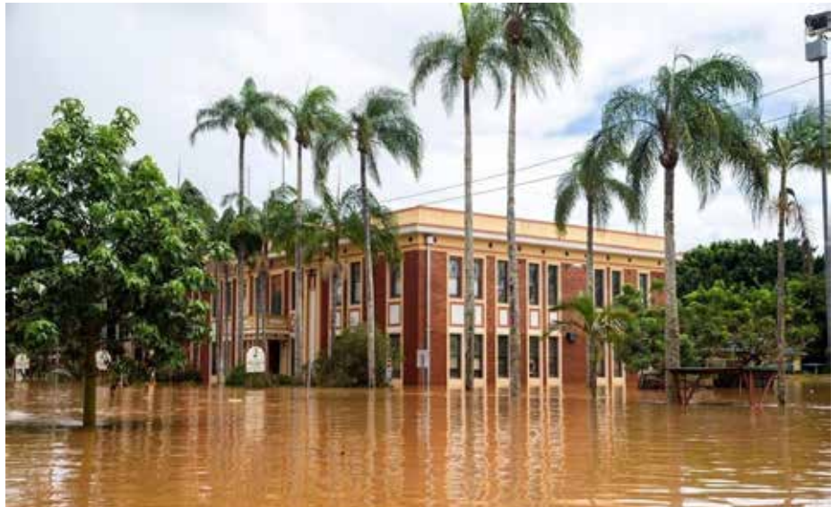
The former Lismore council chambers, now home to Richmond Rivers Historical Society museum, faced extensive repairs and renovations after the 2022 floods. Image: Brendan Beirne.
